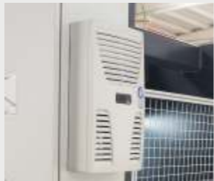
Electrical Cabinet AC Cooling System
